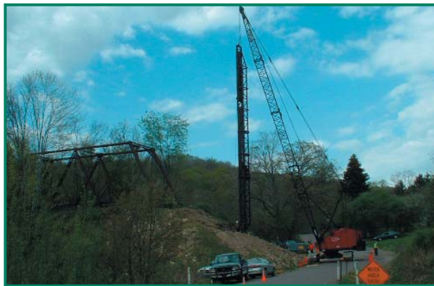
Bollman Bridge shown resting on trail waiting to span Scratch Hill Road while crane drives piles for bridge abutments.
